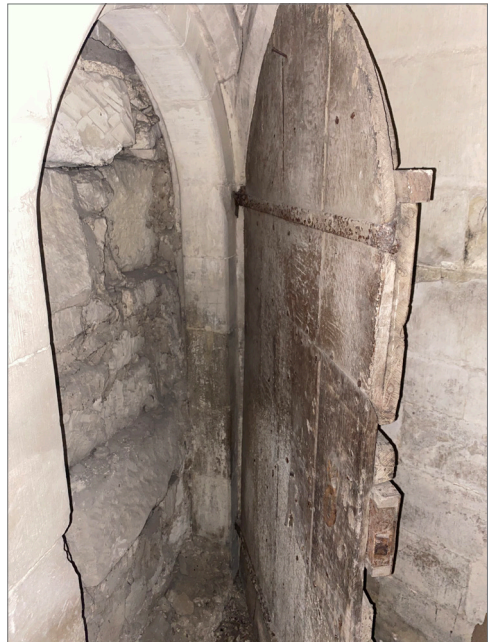
Top: North East Transept stair turret from outside Above: Sealed doorway at base of staircase
