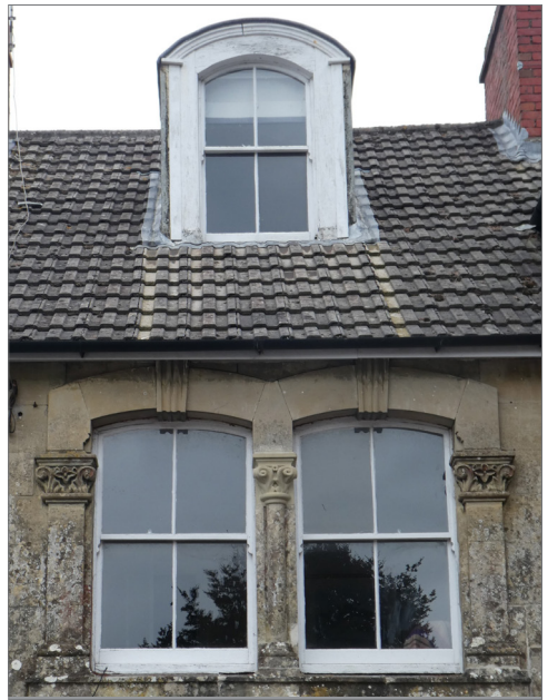
The nextdoor property showing the lost windows as they were
