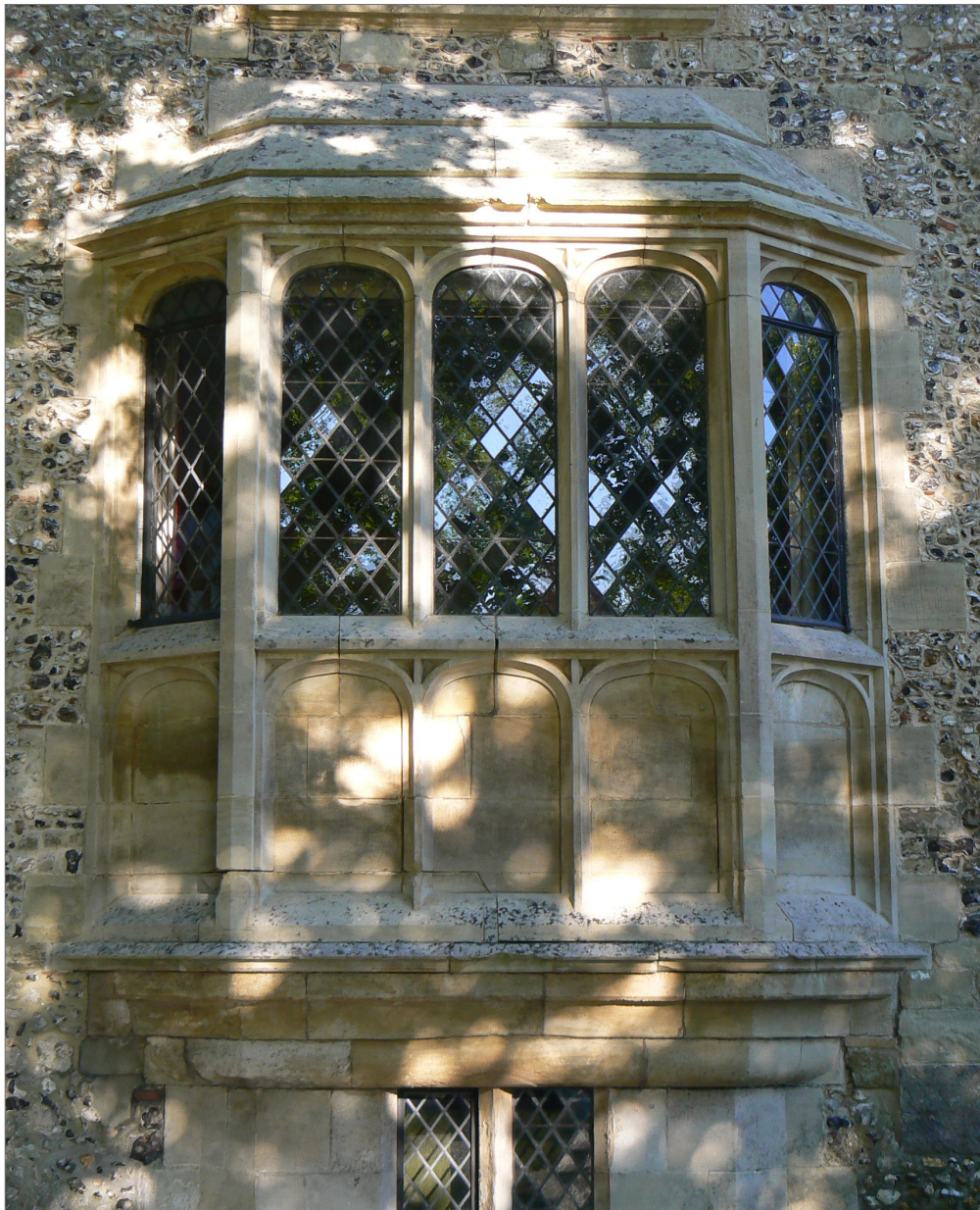
Oriel window at the North Canopy, in the Cathedral Close (see p.16)
